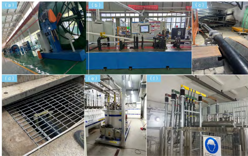
Figure 26. Landmark pictures of Shenzhen superconducting cable demonstration project. (a) Automated production line for concentric HTS cable cores. (b) Continuous welding and encapsulation production line for HTS cable core and cryogenic pipes. (c) Installed HTS cable in the cable tray. (d) Installed HTS cable in the cable trench. (e) Cryogenic refrigeration system. (f) HTS terminal in Binhe Substation.
